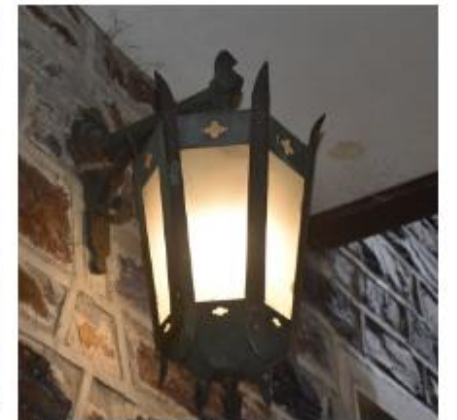
Copper exterior lighting.
