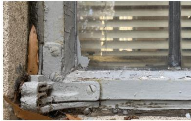
Detail of paint buildup at typical outswing hinge and failing glazing putty.
