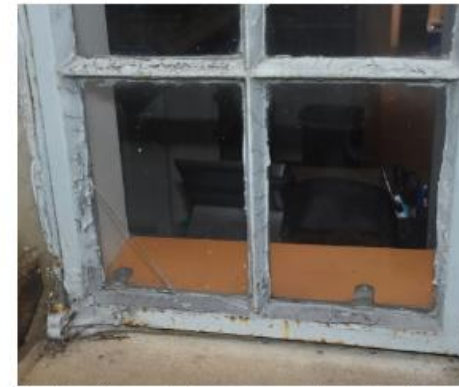
Visible surface rust, failing perimeter sealant and broken pane.
