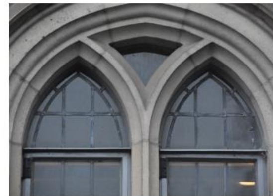
Damaged comes at Gothic arch transom.
