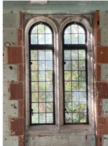
Interior stone surround with minor water staining.
